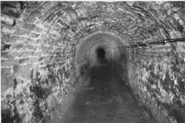
Gunnite mortar finished section of the Victoria tunnel to try and reduce water penetration.
